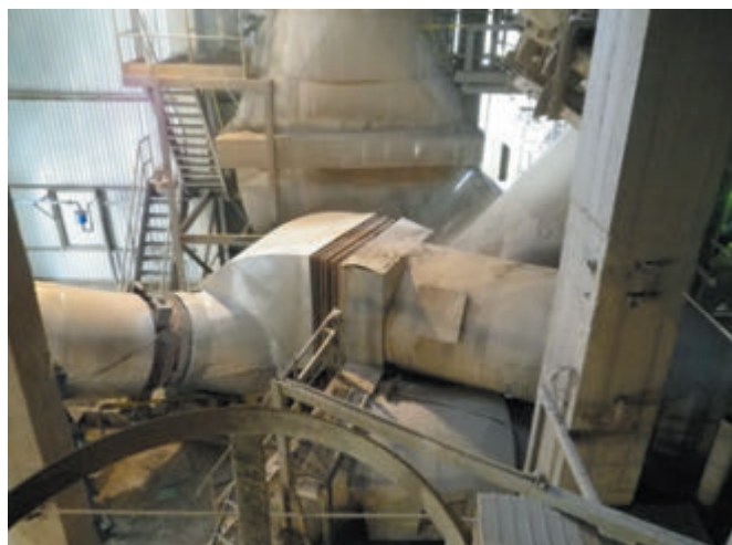
Fig. 2. Real condition on site – gasses distribution
